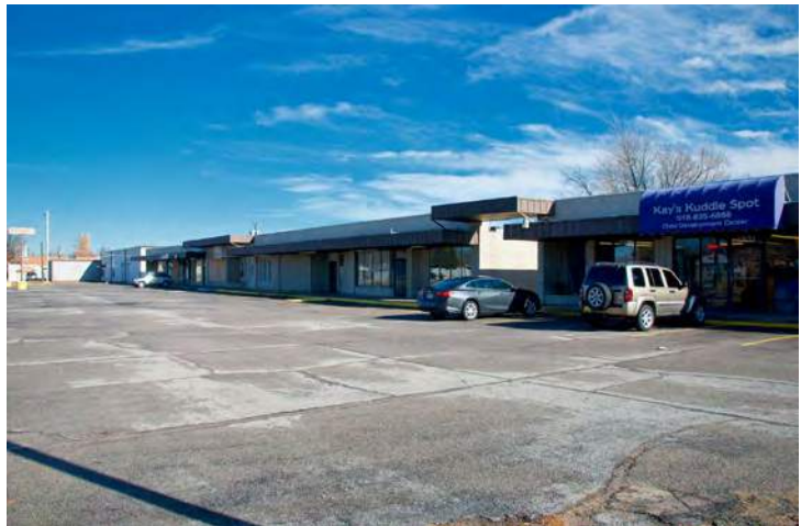
The strip center in the 1200 block of Sheridan Avenue is one of several area properties in need of significant maintenance and repair.
