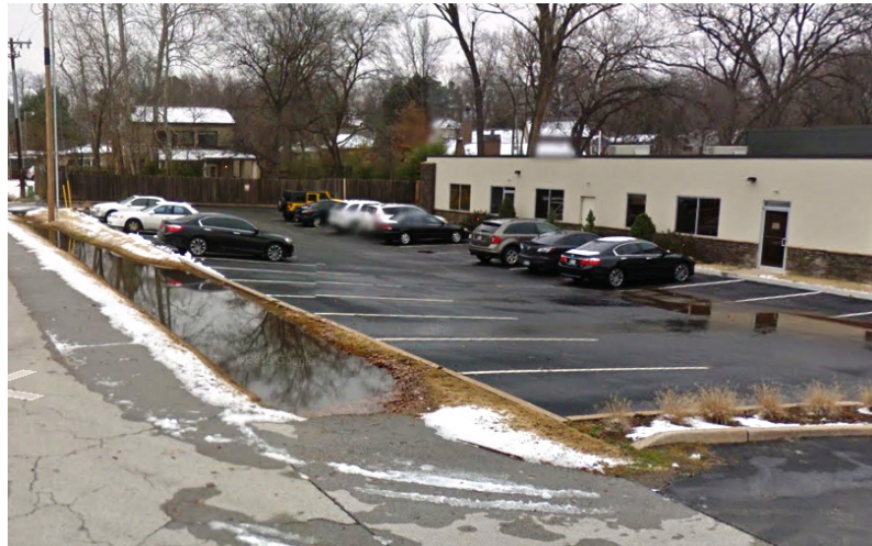
Clogged bar ditches, below street level construction and slab-on-grade buildings contribute to flooding in RLA #59.
