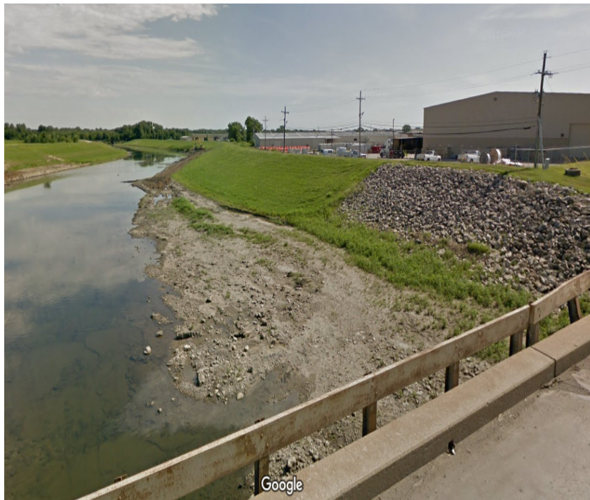
Looking north on Mingo Creek from the E. Pine St. bridge. RLA #50 is at the right, behind the levee.
