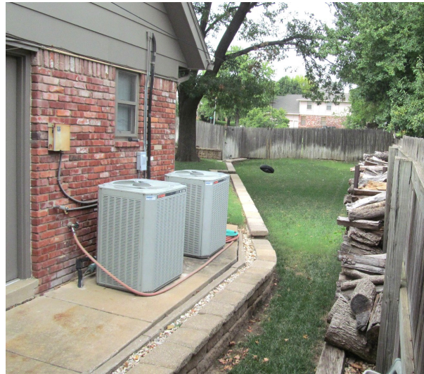
This platform and wall protect the home and air conditioning equipment from shallow flooding.
