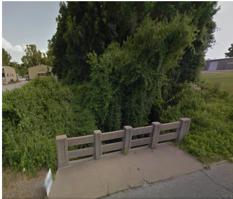
Looking south on Mill Creek from E. 11 th St. On the south side of 11 th St. Mill Creek flows in an open channel. North of 11 th St. the stream is carried in storm sewers to McClure Park.
