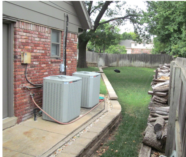
This platform and wall protect the home and air conditioning equipment from shallow flooding.
