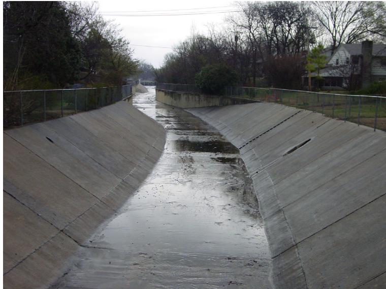
Little Joe Creek channel near E. 53 rd St. and S. Toledo Ave., looking east--upstream)
