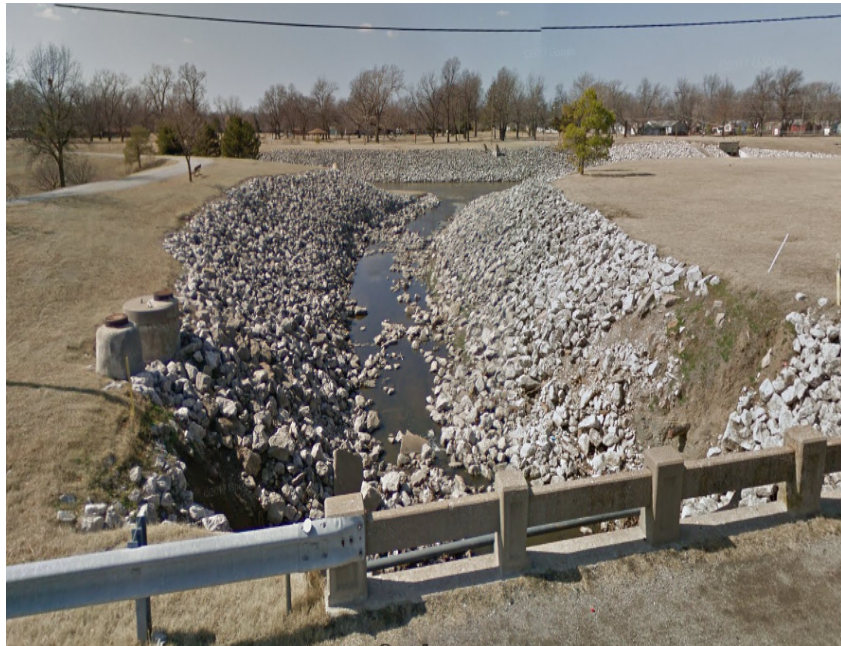
Tupelo Creek, looking downstream from the Mingo Rd. bridge between E. 5 th and E. 5 th Pl. to the junction with Mingo Creek.
