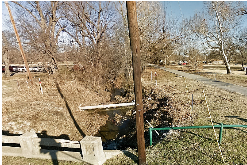
Parkview Creek at N. 41 st W. Ave. and the Katy Trail, looking east.
