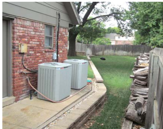
This platform and wall protect the home and air conditioning equipment from shallow flooding.
